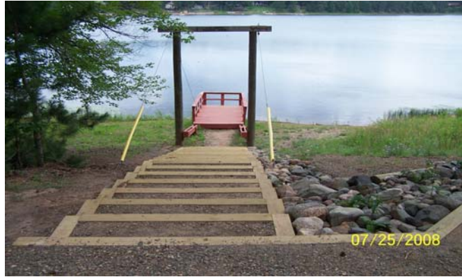
ABOVE: Looking down the newly installed steps to the fishing pier at Runkle Lake.
