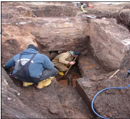
City employees John Lortie & Gerard Valesano repair broken water line under foundation.
